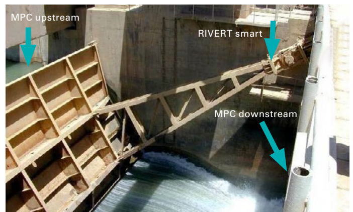
Picture of installation
